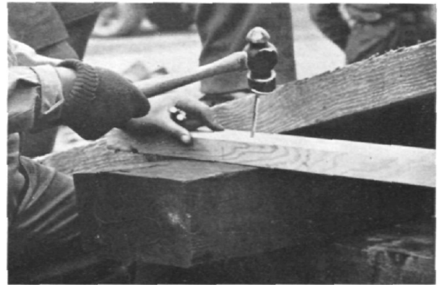
Fig. 4—Cleats keep the boards from spreading out sideways as the heavy trucks roll up.
