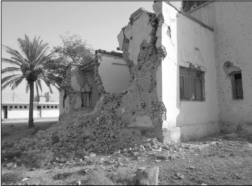
Al Muthenna Intermediate School in Samawah in southern Iraq was damaged when Iraqi troops took shelter in the school. (Photo by Thomas Hartwell)
